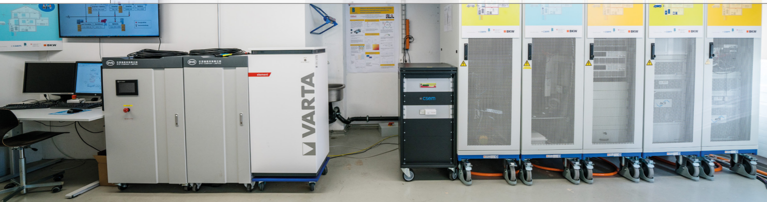
Batteries, emulators, and circuit and control technology for load flow management.
